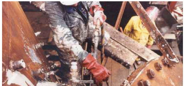
8. Once void is filled, valve is shut off. Material pressure line is then moved to next nipple. Nipple that was just grouted is then capped. Material will flow out adjacent nipples when void is filled.
