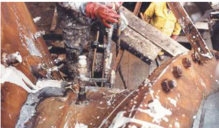
6. Both valves open. Material is flowing in under pressure. Pressure is monitored to not exceed 80 psi. Material used is a mixture of ErgonArmor's HB™ and CORLOK™ B Mortars.
